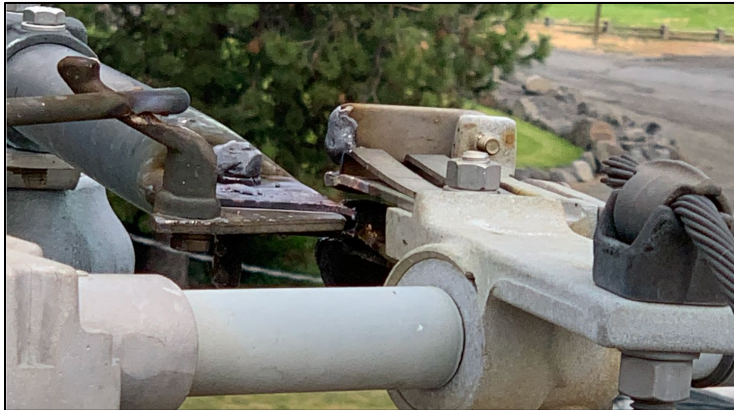
Figure 1. Damaged line switch
