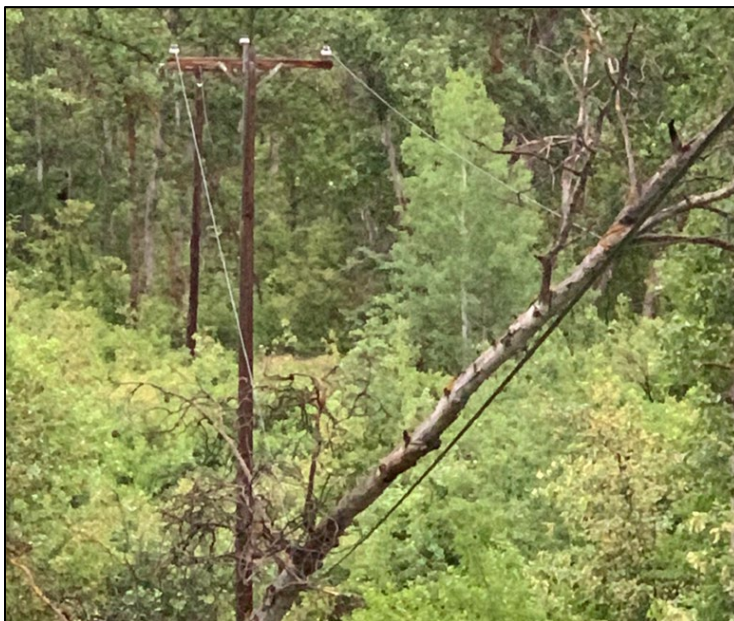
Figure 2. Tree down fault
