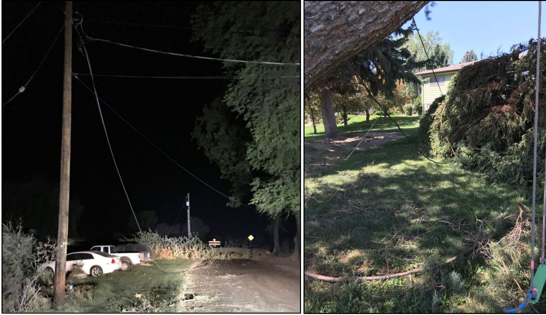
Photos of damaged equipment from downed trees.
